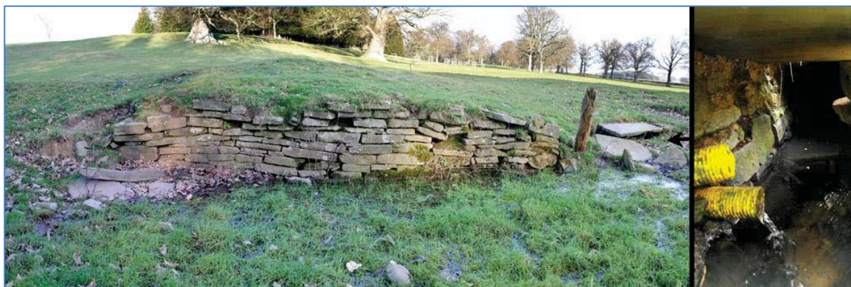
Stone wall abutment to pond in Little Park fed by the culvert (right) that runs from the Meres to the Wye. See map 18 below for the full course of the culvert. Note the modern drains that run into the culvert at this point. See section 9.1 for recommendations.
