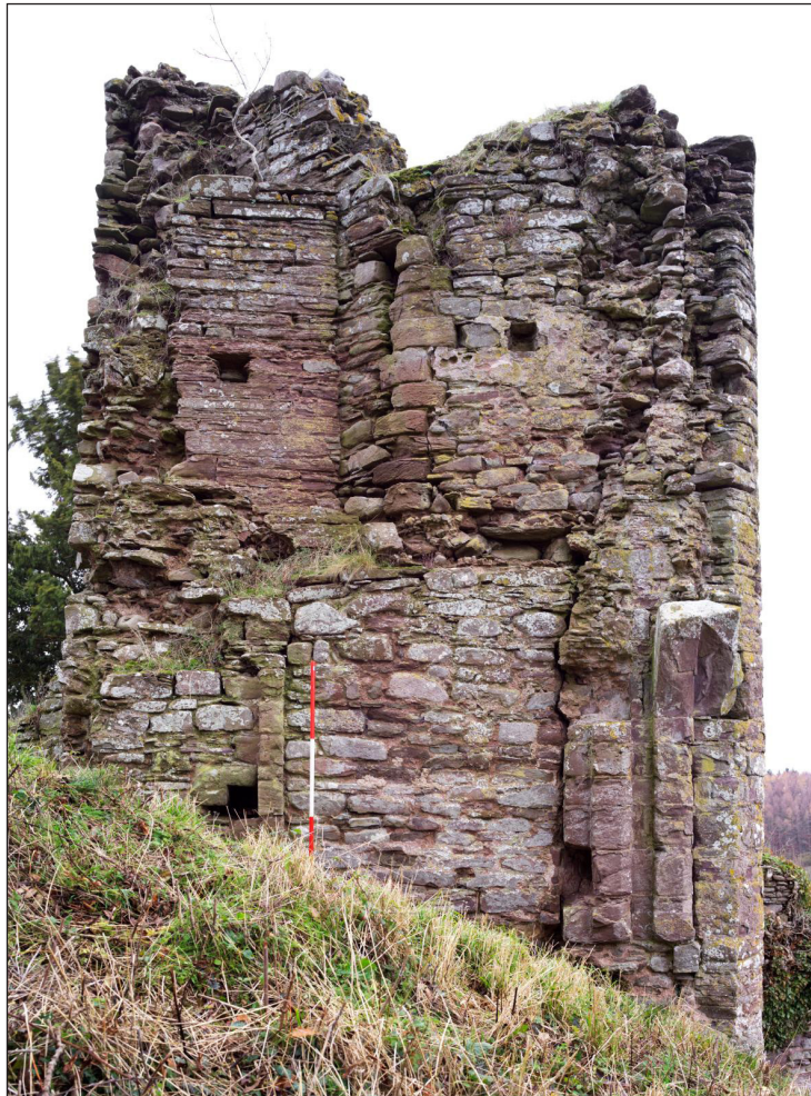
Figure 10 Southwest corner of the tower, interior, showing the surviving western opening at first-floor level (DP195367).
